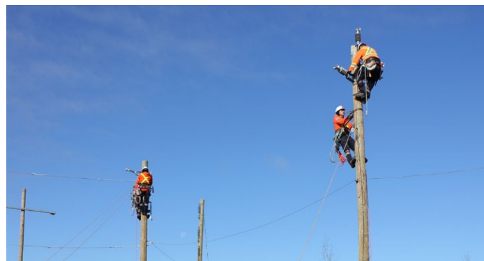
■ The fourth round of Line Crew Ground Support Training for the Wataynikaneyap Power Project
