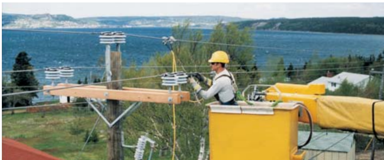
Investment in capital initiatives helps control costs and enhances reliability of service to customers.
