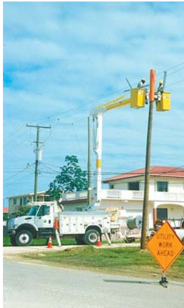
A commitment to employee and public safety is integral to Belize Electricity's daily operations.
