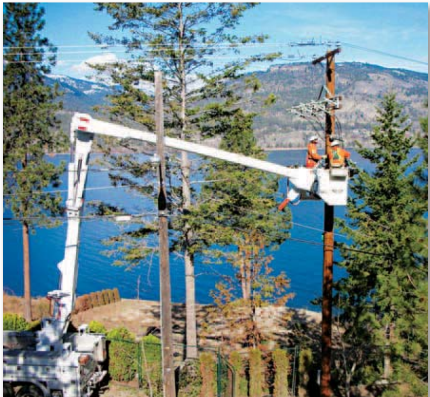
FortisBC's utility assets include more than 6,750 kilometres of transmission and distribution power lines and four hydroelectric generating plants with a combined capacity of 235 MW.
