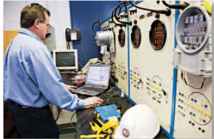
FortisOntario customers continue to rate reliability/safe delivery of electricity and quality of service high priorities at 94 per cent and 87 per cent, respectively, in 2006.
